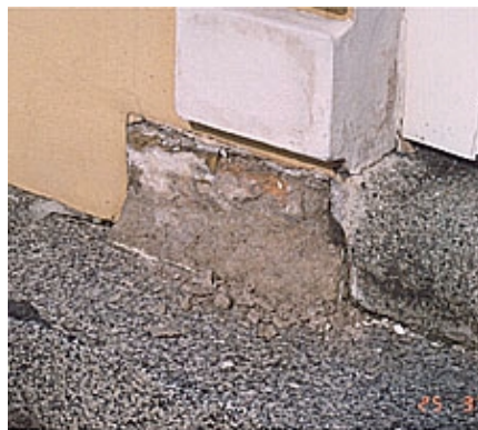
Damaged render left to the entrance before refurbishment work started
