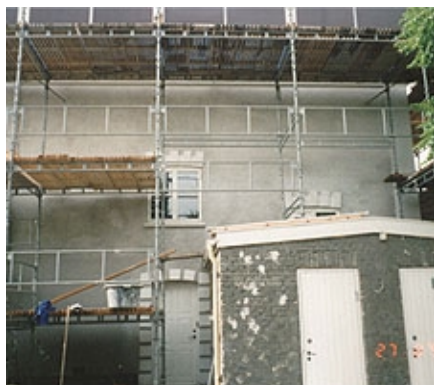
Right side of the building treated with VANDEX REFURBISHMENT PLASTER white as finish before painted
