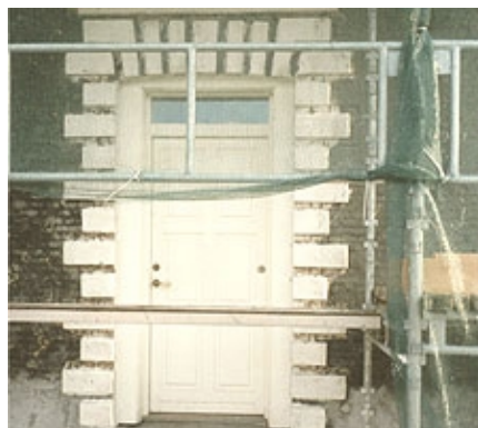
Entrance, lower part treated with VANDEX BB 75 and upper part with VANDEX ROUGH CAST
