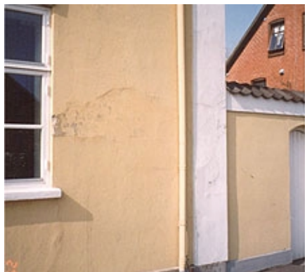
Damaged cracked corner at the front before refurbishment work started
