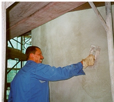
Skilled workmanship by hand is a very important part of the final result
