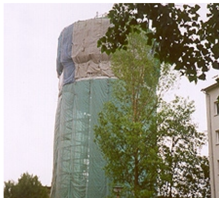
The tower was totally covered in order to provide protection for the refurbishment work
