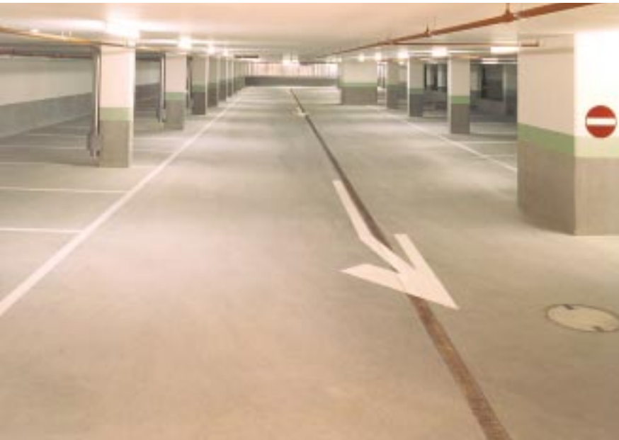
Figure 1: Overview of the finished car park with a cementitious waterproofing screed on the floor.
