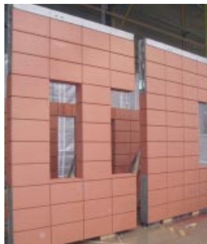
Figure 4: Interlocking precast terracotta panels with cross-flow ventilation apertures that are a feature throughout the ground floor.
